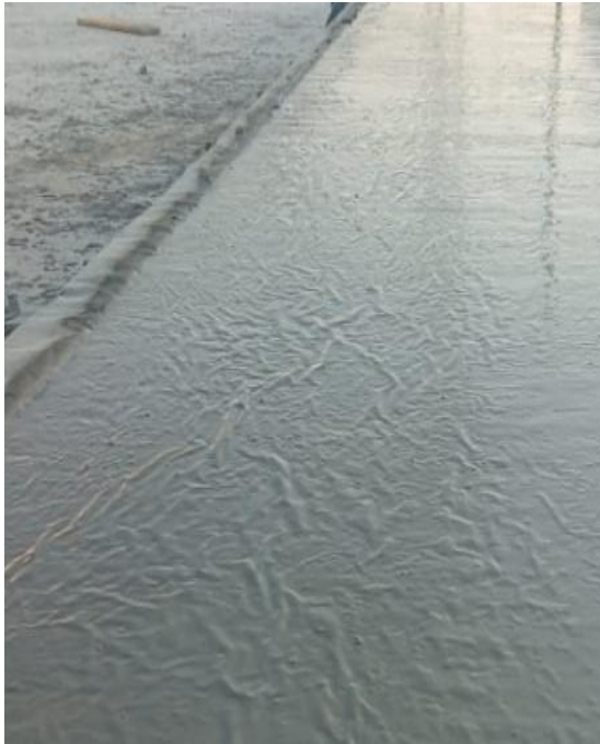
Fig 3 Rippled a poor condition
