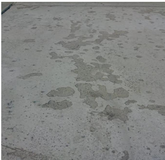
Fig 5 New Placed Concrete turned to long
